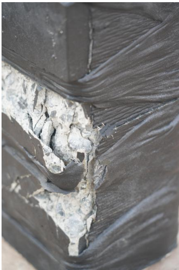
a) Fiber rupture
