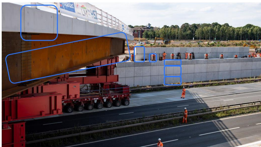
Figure 3. Offsite Manufactured modular bridge constructed in the UK using the DFMA approach and installed by SPMTs (New Civil Engineer, 2020)
