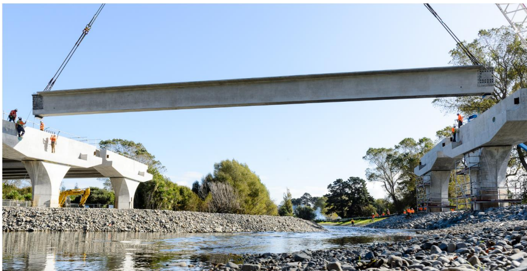
Figure 2. Offsite Manufacture of prestressed super tee girders and pier cross heads on the MacKays to Peka Peka Expressway (M2PP) project, 2017, Beca, New Zealand.
